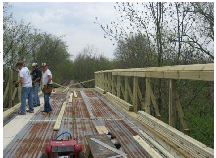
Led by Harry Denham, members of the Friends of the Nickel Plate (and Club Kokomo) work on the first 50 foot section of the bridge over Pipe Creek.
